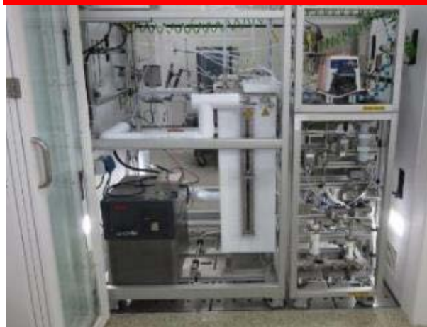
Plug Flow Reactor Skid
